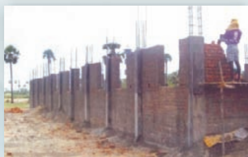
VILLAGE INTO SMILES as a SCHOOL is being built at Pulikat village
